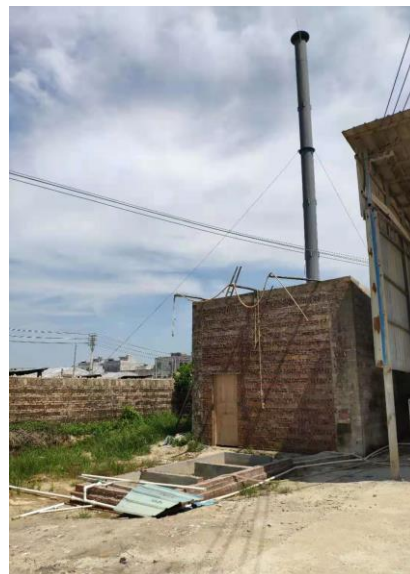
喷淋室及 15m 排气筒
